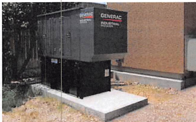
Motorola Alternative Building 10x12 foot with an optional outdoor generator based on the selected equipment load configuration.
