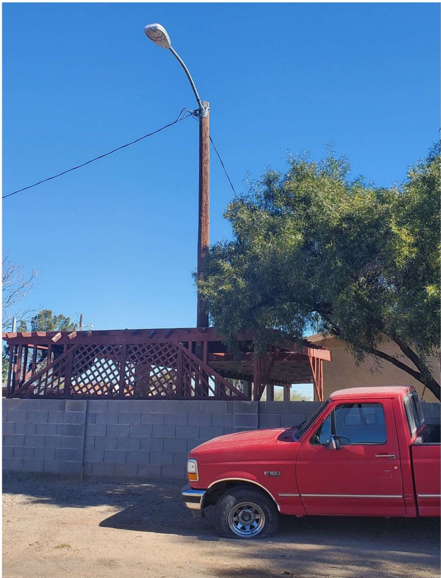
FIGURE 3.2. EXISTING LIGHT POLES
