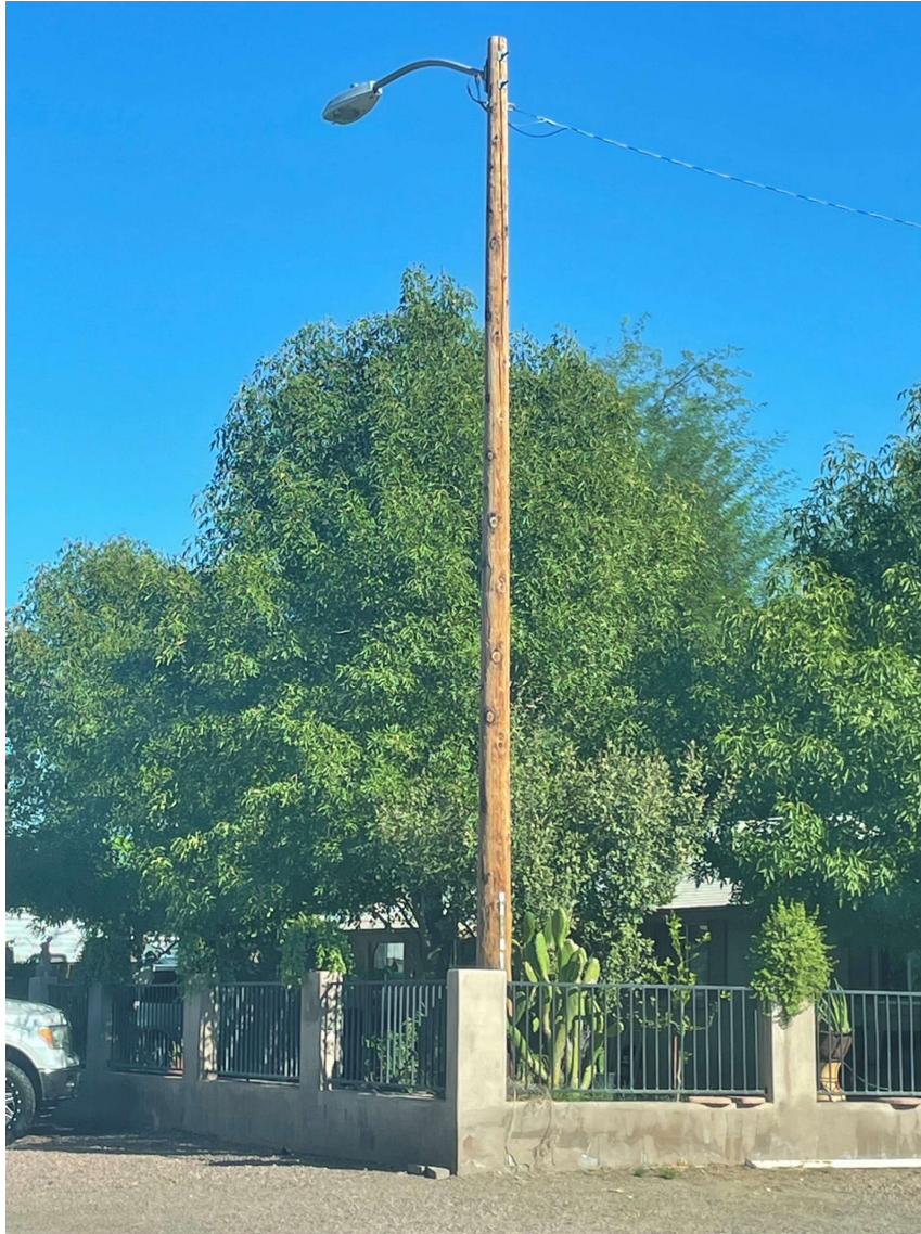
FIGURE 3.1. EXISTING LIGHT POLES
