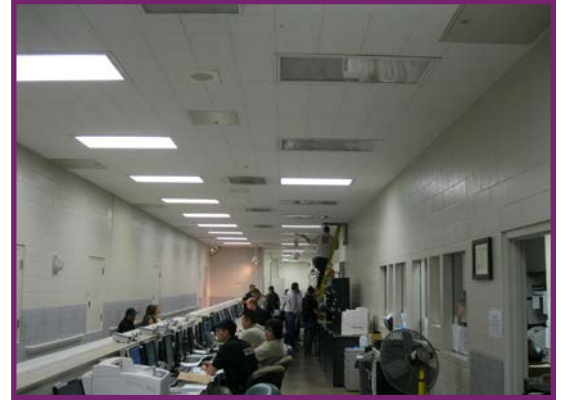
Maricopa County JOC - 4th Avenue Jail HVAC Upgrades
