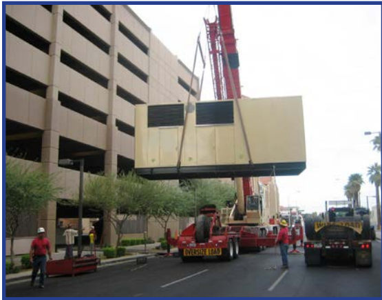
Chandler Data Center
