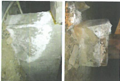
These images show the effects of sulfate attack on a shallow foundation and grade beam.
