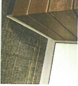
This detail shows several different trades coming together in one location, which can be difficult to execute in the field. In such cases, we would recommend stand-alone or in-place mock-ups to demonstrate the proper quality expectations.
