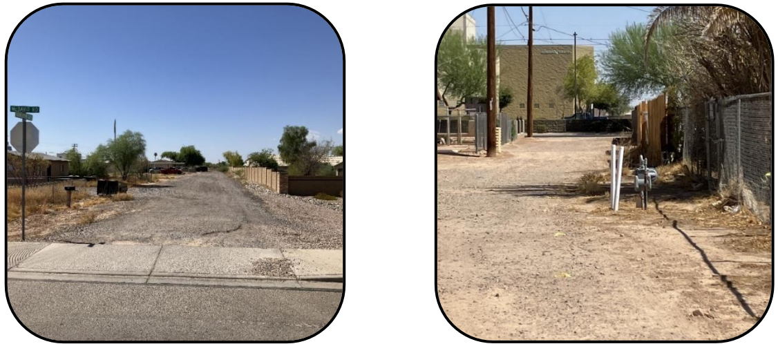
Figure 9: Unpaved Alleys and Streets
